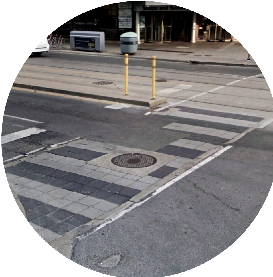
Inconsistent and poorly maintained crosswalks
