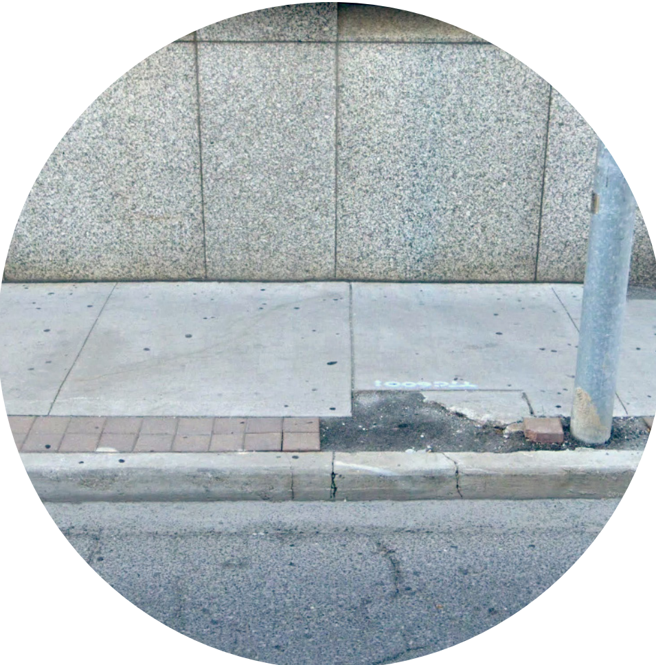
Inconsistent and poorly maintained paving
