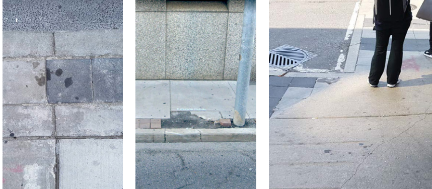
Today, sidewalks of inconsistent materials with multiple joints have deteriorated over time
